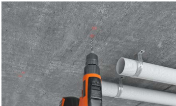
The diffuser is fixed to the concrete ceiling before gypsum board framing is installed.
